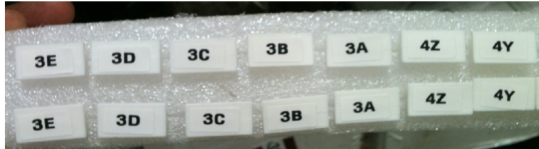
Figure 5: Example Power Cable Labels
