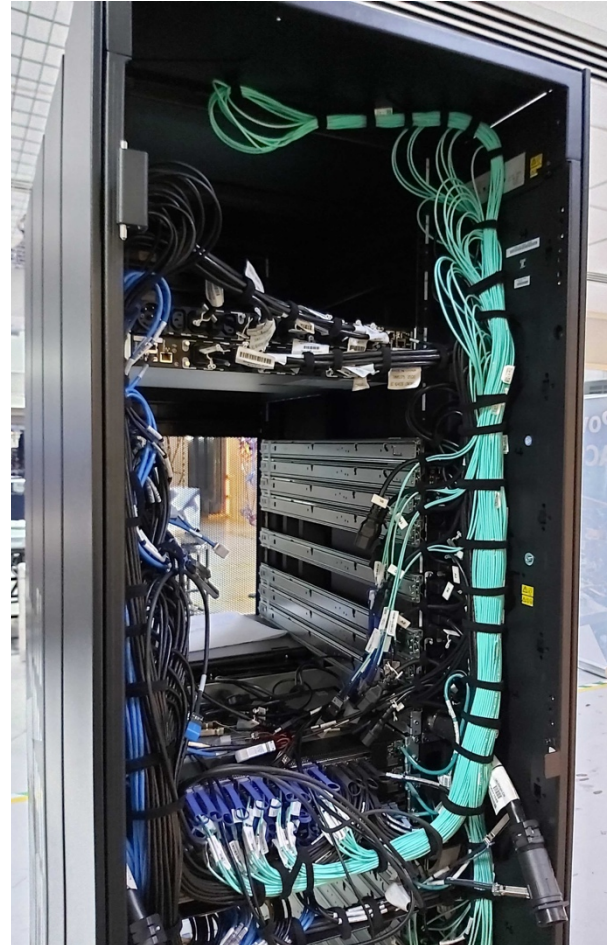
Figure 2: Rear view of an IBM Spectrum Fusion HCI rack
